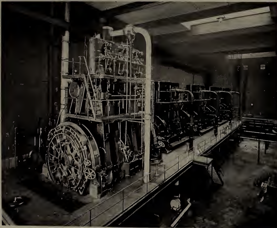
VIEW IN THE PLANT OF THE EDISON ELECTRIC ILLUMINATING COMPANY OF BOSTON, Atlantic Avenue, foot of Pearl Street.
